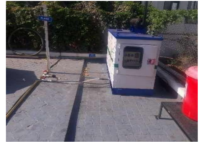
Use of Bio-methane for electricity generation
