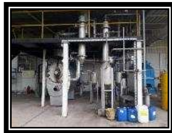
Installed and commissioned “Waste plastic to Fuel Conversion plant” with a yield of almost 70%.
